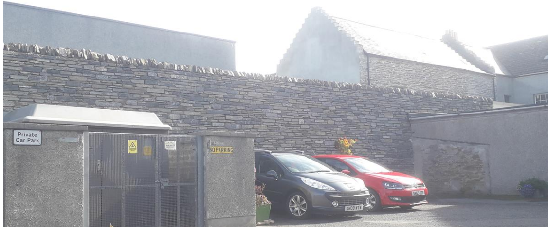
New stone boundary wall, screening flat roofed extension. Building now visible, and re-pointed, to rear of image
