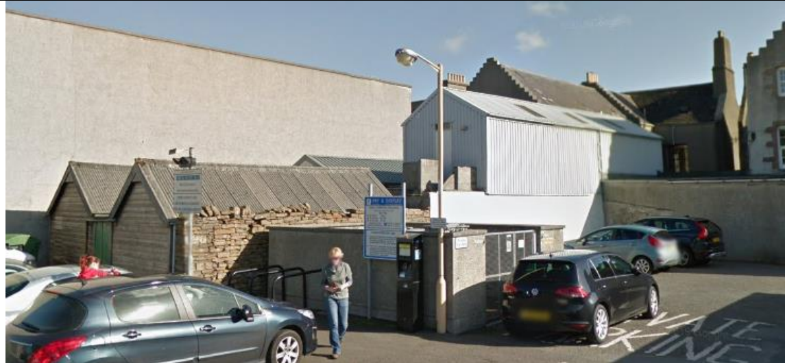
Yard to rear of building before works, showing boundary wall in poor condition and building (with chimney stacks) obscured
