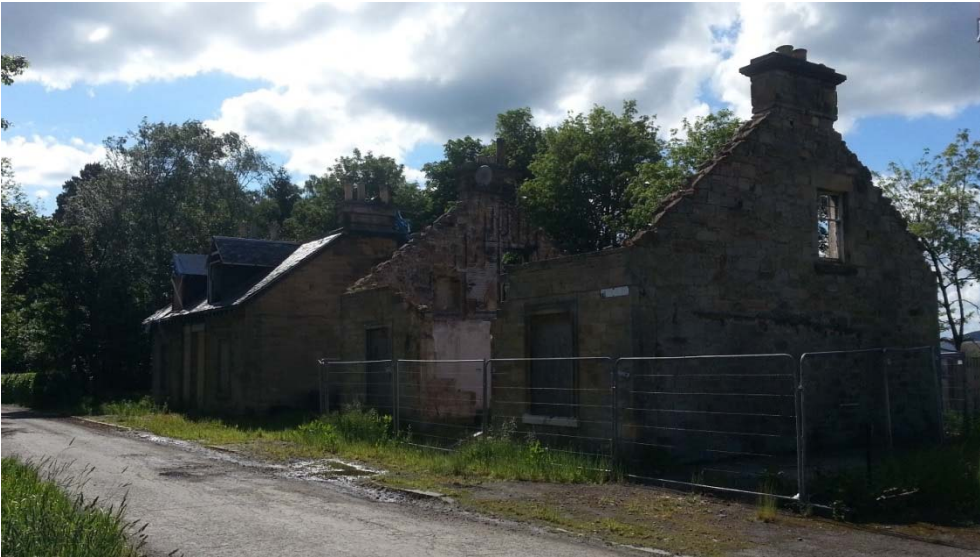
Buildings which will be converted into housing as part of the Rosslinlee development.
